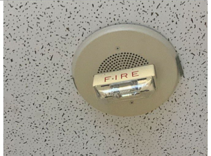
26 - FIRE ALARM SYSTEM
