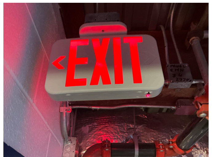
30 - EMERGENCY & EXIT LIGHTING SYSTEM
