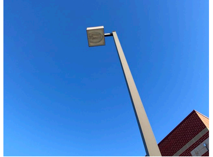
38 - PARKING AREA LIGHTING
