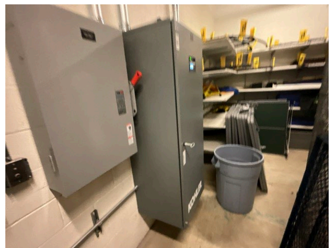
24 - AUTOMATIC TRANSFER SWITCH
