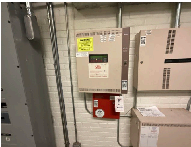
27 - FIRE ALARM PANEL
