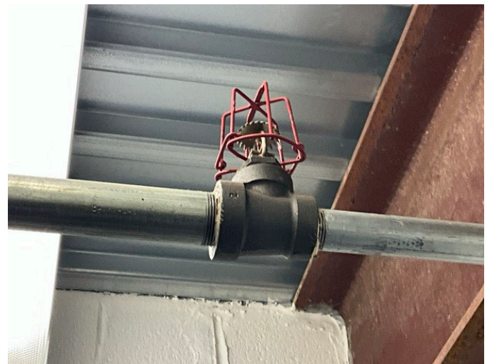
28 - FIRE SUPPRESSION SYSTEM
